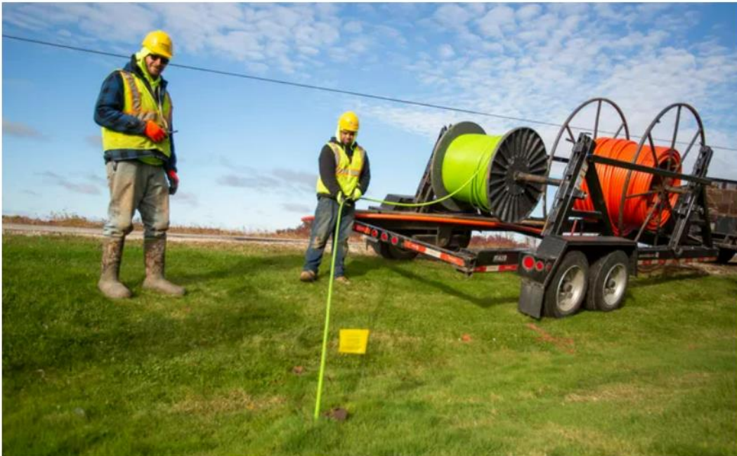
While construction employee Nathan Braaksma, left, watches, Tony Galdan threads special conduit that will eventually house a fiber optic cable which will bring internet to rural Fond du Lac county, Tuesday, Oct. 18, 2022, in Fond du Lac Wis. Gary C. Klein/USA TODAY NETWORK-Wisconsin
