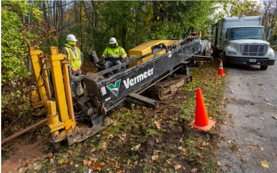
A directional drill bores into the earth by White Construction's Logan Miller, left, and Lanell Brown, Tuesday, October 18, 2022, in Fond du Lac, Wis. The drilling is part of the process of placing fiber optic cable underground so that rural areas will gain access to fast internet. Gary C. Klein/USA TODAY NETWORK-Wisconsin
